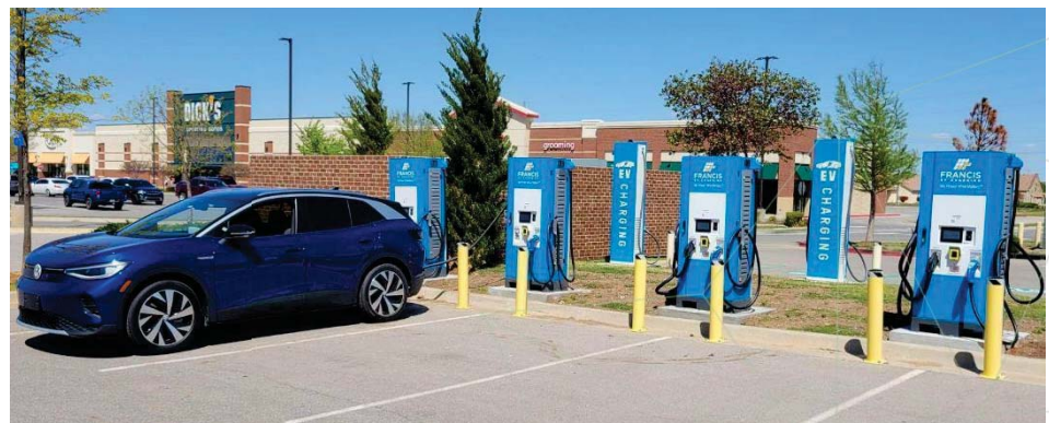
Public Charging, Oklahoma Francis Energy 120 Ports DCFC
