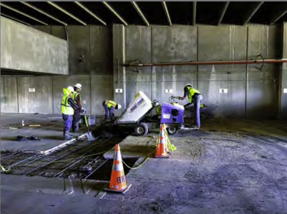
GSA - Replacement of Domestic Water & Sanitary Waste Lines at RC White Building - El Paso, TX
