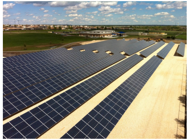
Liberty Village Fort Hood – 682 kW
